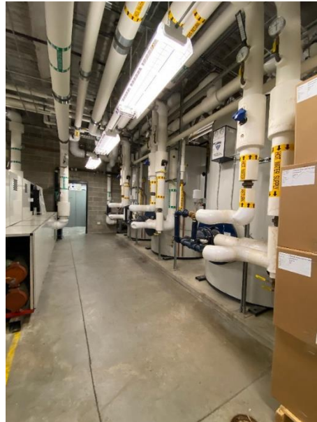
Fig. 16: Domestic water storage system.
