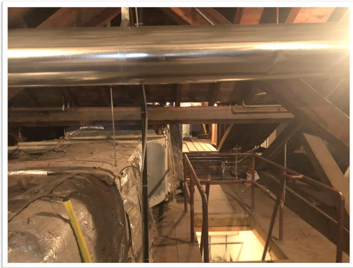
Fig. 3: County Hall attic showing air handler.
