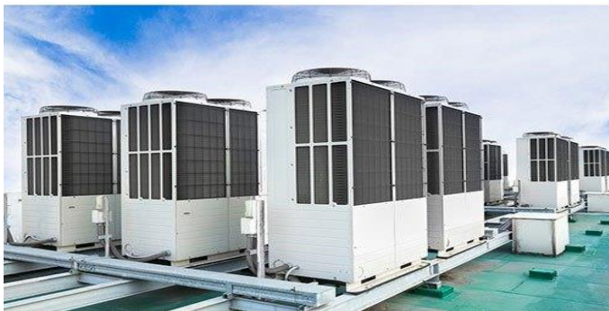
Fig. 11: Roof mounted VRV heat pump system.
