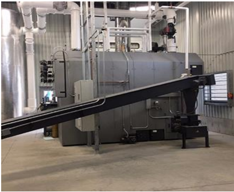
Fig. 7: Typical Woodchip Boiler.
