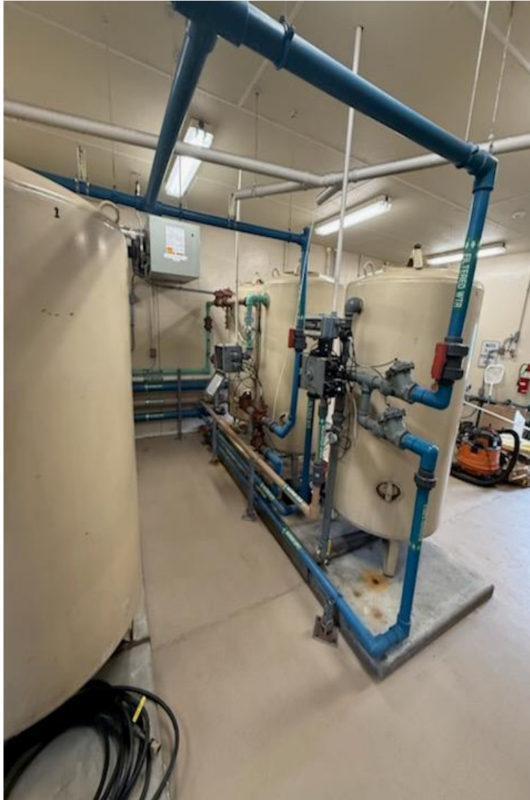
Secondary Filter Trane Photo by Aaron Newman, March 2026
