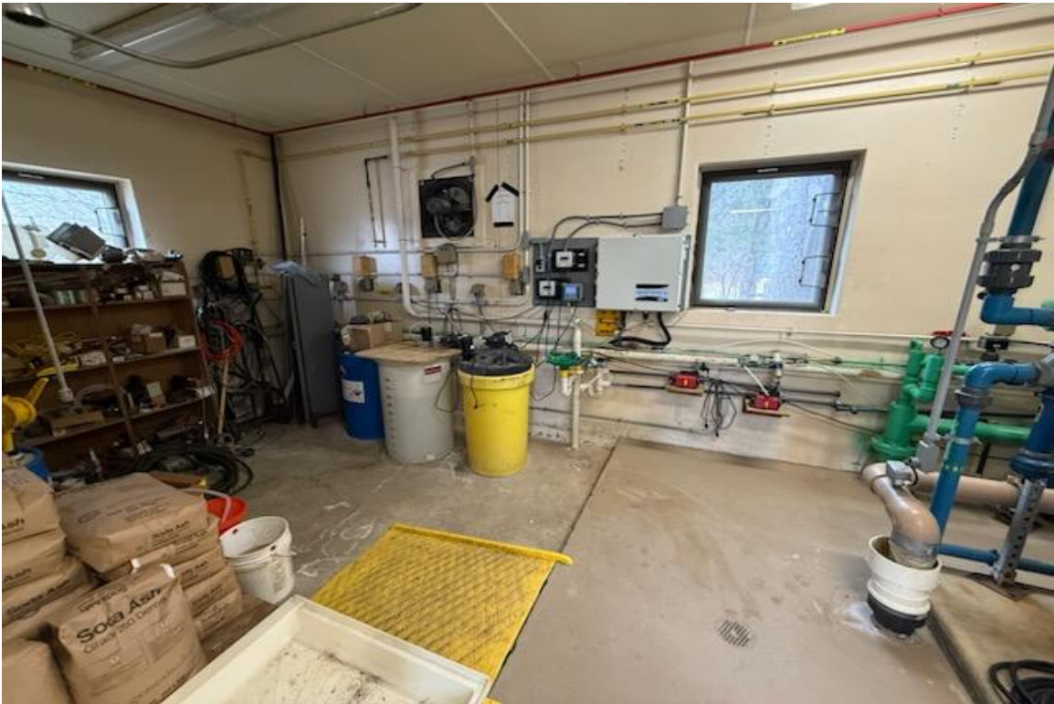
Raw Water Chemical Injection System Photo by Aaron Newman, March 2026
