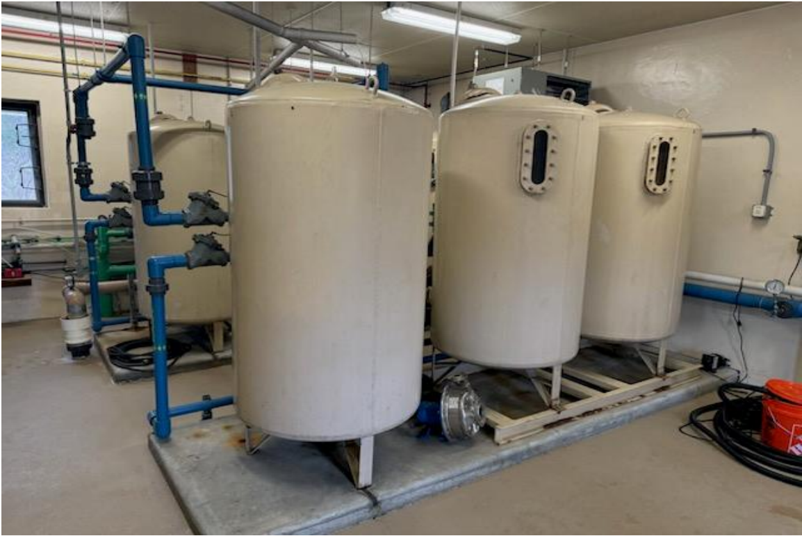
Carbon and sediment Filter Trane Photo by Aaron Newman, March 2026
