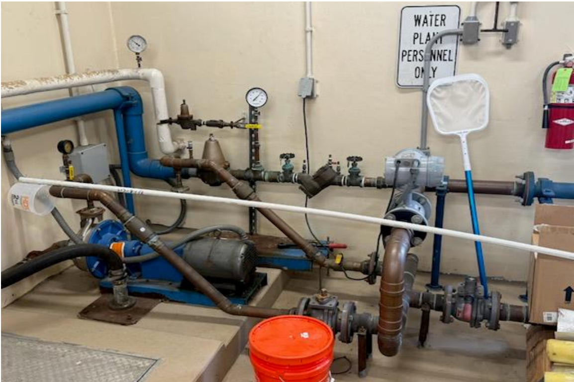
Clear Well and Pumping Station to Distribution System Photo by Aaron Newman, March 2026
