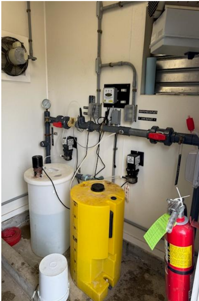
Well Pump House and Chemical Injection Photo by Aaron Newman, March 2026
