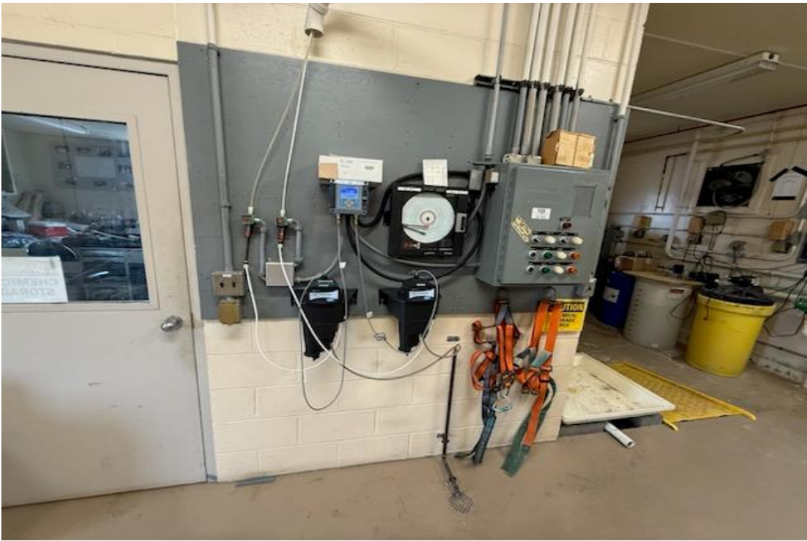
Control System and Data Logging. Photo by Aaron Newman, March 2026
